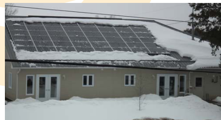
SOLAR PV INSTALLED ON THE TENNISCO MANOR ASSISTED LIVING FACILITY
