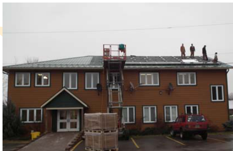
SOLAR PV PANELS INSTALLED ON A LOCAL ADMINISTRATION BUILDING
